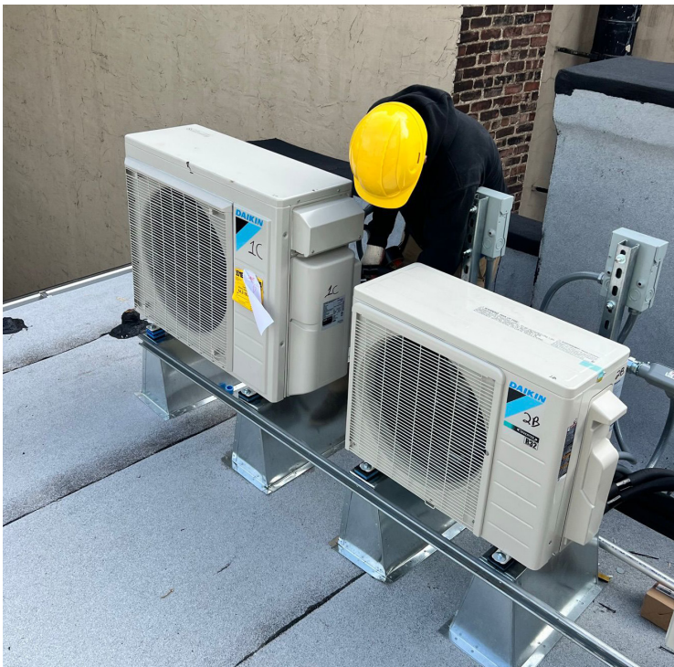
An Energy Plus technician installs advanced energy equipment on a New York City rooftop.
