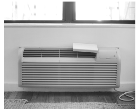
Typical PTAC (interior view)
