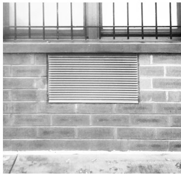
Typical Sleeve AC (exterior view)
