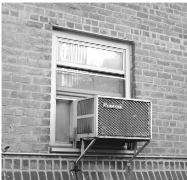
Typical Window AC (exterior view)
