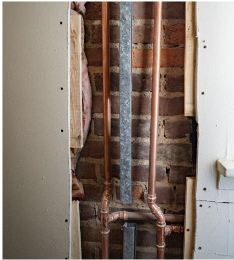
A new two-pipe hydronic heating system transports hot water more efficiently throughout the building.
