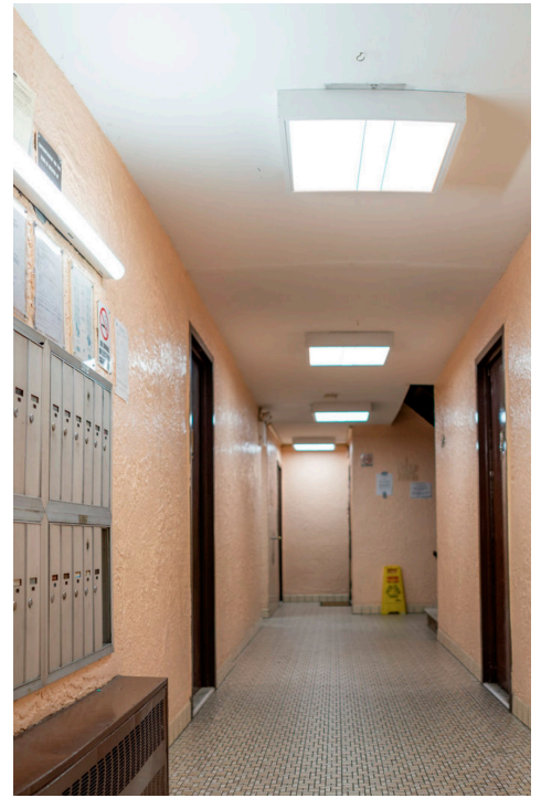
LED and elevator upgrades in common areas reduce electric and maintenance costs.
