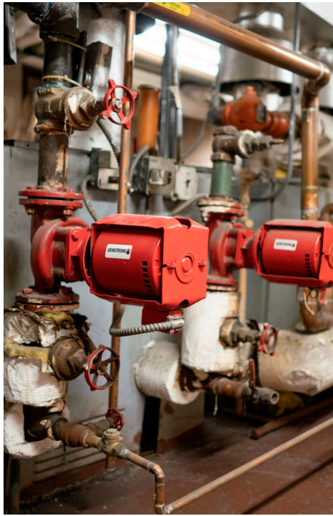
High-efficiency domestic hot water heaters reduce emissions to comply with Local Law 97.
