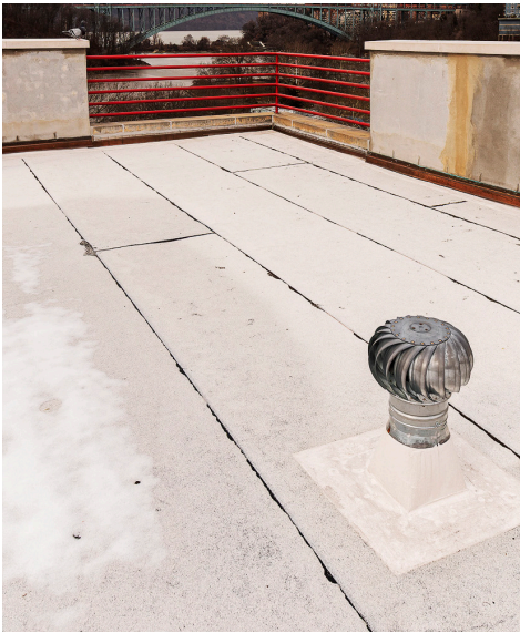
New roof with enhanced insulation and greater reflectivity helps maintain consistent indoor temperatures and prevents heat transfer.
