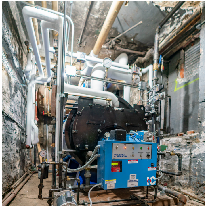
A new boiler increases efficiency and reduces carbon emissions.
